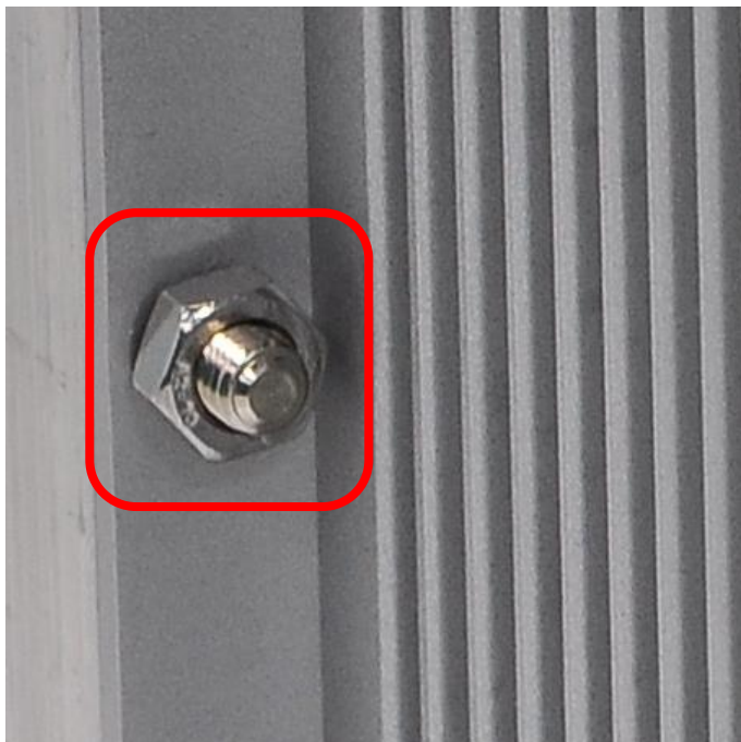
Ground screw of the switch
